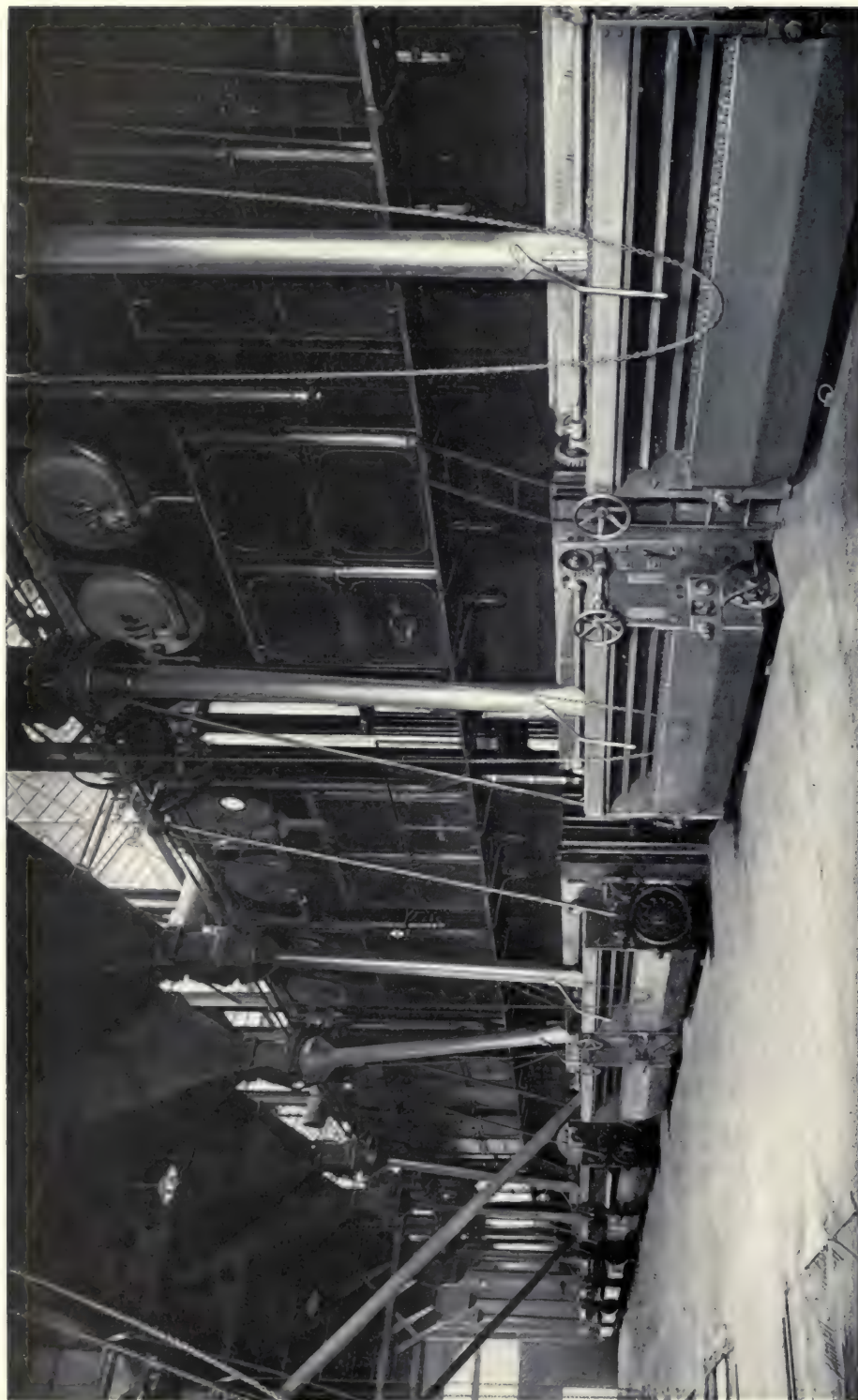
PUBLIC SERVICE CO. OF NORTHERN ILLINOIS, BLUE ISLAND, ILL., PLANT. BABCOCK & WILCOX SUPERHEATERS INSTALLED IN 9600 HORSE POWER OF BABCOCK & WILCOX BOILERS AT THIS STATION. THIS COMPANY HAS BABCOCK & WILCOX SUPERHEATERS INSTALLED IN 12,600 HORSE POWER OF BOILERS IN ITS VARIOUS STATIONS
